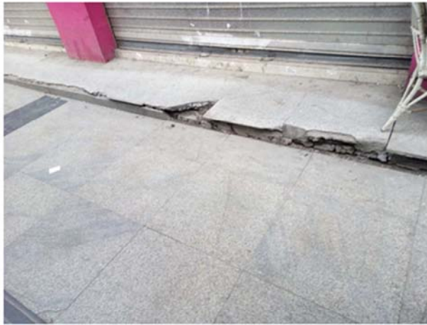
(a) Surface subsidence and crack
