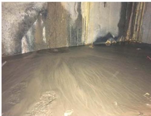
(c) Sand gushing from floor
