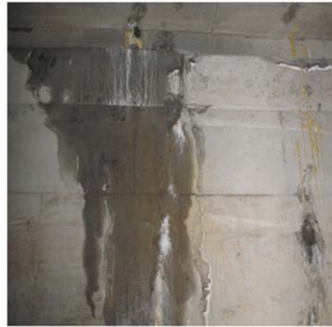
(b) Seepage of sidewall
